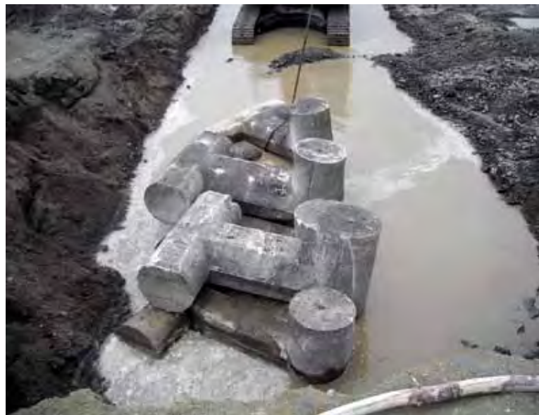
Above: Dolosse are placed on top of one another to form an interlocking wall.
